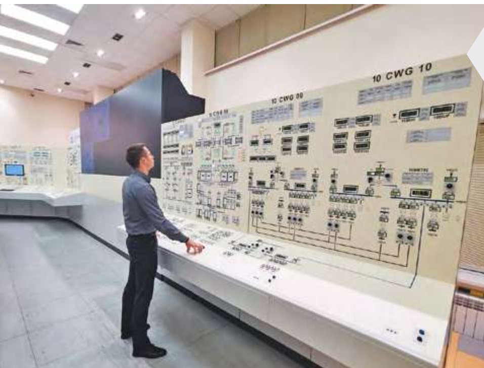
Training on the full-scope simulator of the MCR of the NPP with the VVER-1200 reactor. Novovoronezh NPP. 2019
