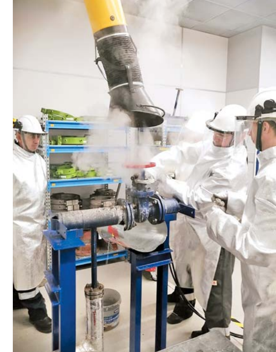
Only a highly qualified specialist can locate the leak without stopping the equipment
